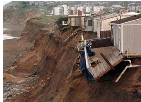
Homes built on a cliff near Pacifica, California collapse as ocean waves erode the cliff.
